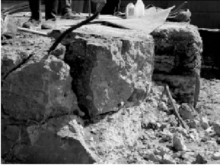
FIG. VI-4. Breaking of the mass concrete roof of repository No. 2 with an electric discharge unit.
