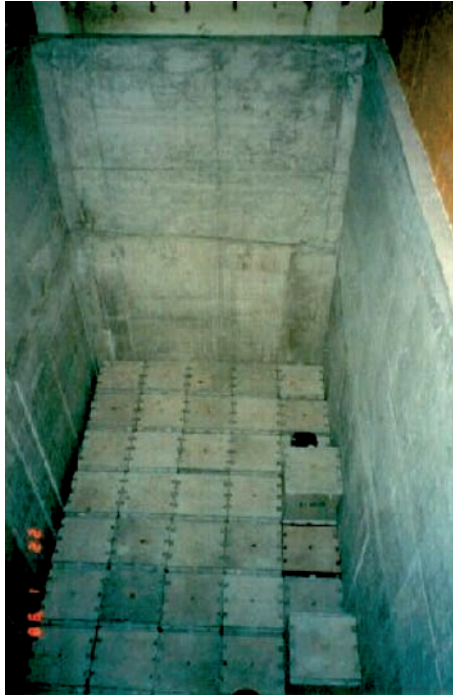
FIG. II-6. Interim store for conditioned solid waste at Paldiski.
