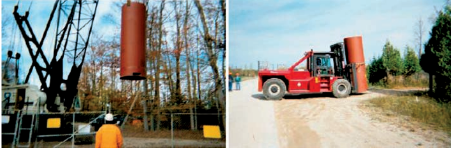
FIG. 8. Lifting a 25 t encapsulated ILW container with a conventional crane and forklift truck.
