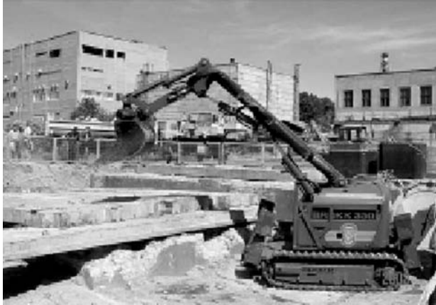
FIG. VI-6. Radioactive waste extraction with robotics equipment.
